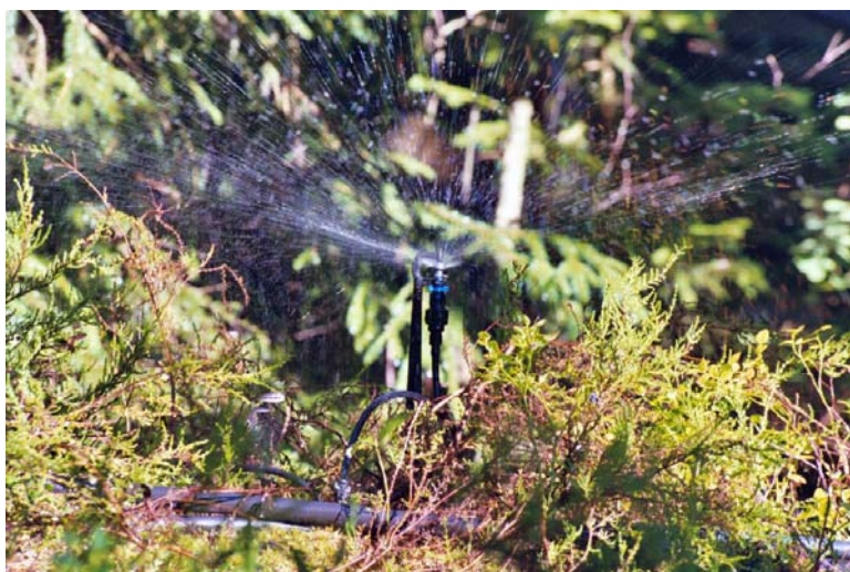
Figure 3. One of the 242 sprinklers installed at Gårdsjön G1 catchment to simulate heavy rains and sea salt episodes.
